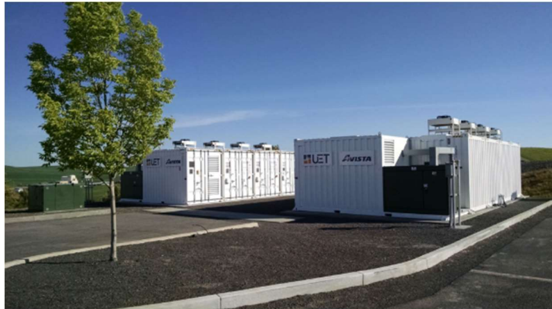
Figure 5.5 A 1 MW / 4 MWh containerized VRFB system installed in Washington (USA) 63
