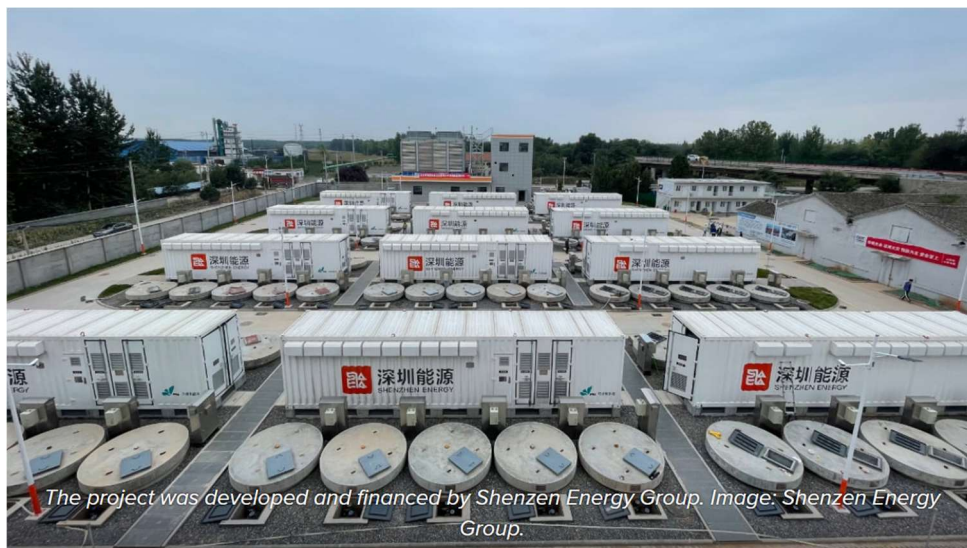
Figure 3.2: A large-scale flywheel energy storage facility (30 MW) in Shanxi, China, consisting of 120 modular flywheel units housed in containers (Shenzhen Energy Group, 2024). Such installations demonstrate the ability to scale FESS by aggregating many modules, each contributing a fraction of the total power and energy 8
