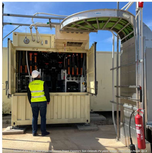
Figure 5.6: The largest vanadium redox flow battery (VRFB) at a solar farm in Europe has been switched on by Enel Green Power in Mallorca, Spain 67
