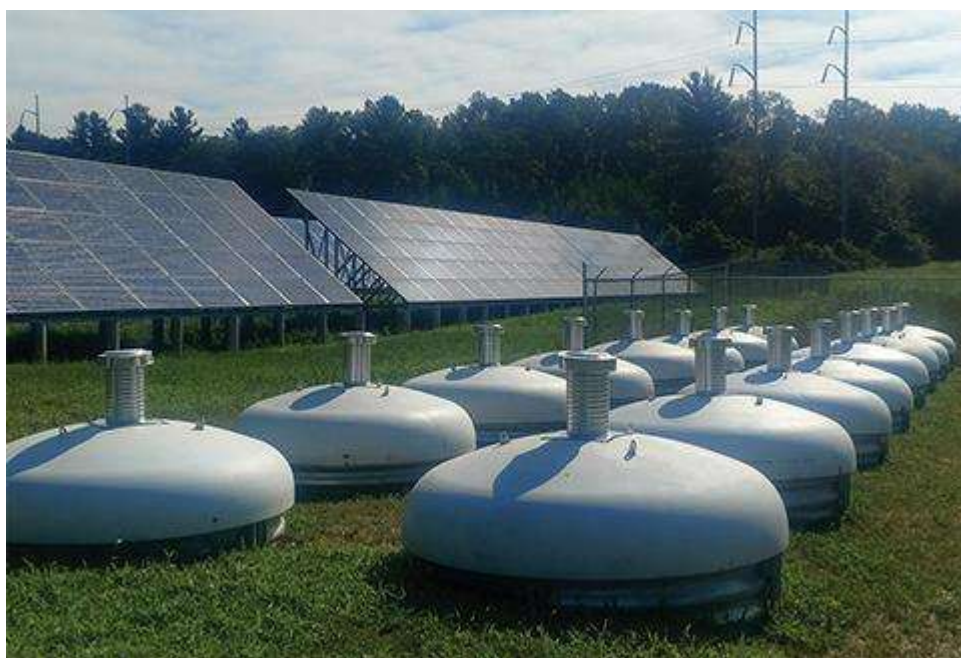
Figure 5.6 West Boylston Municipal Lighting Plant 128kW/512kWh flywheel energy system 127
