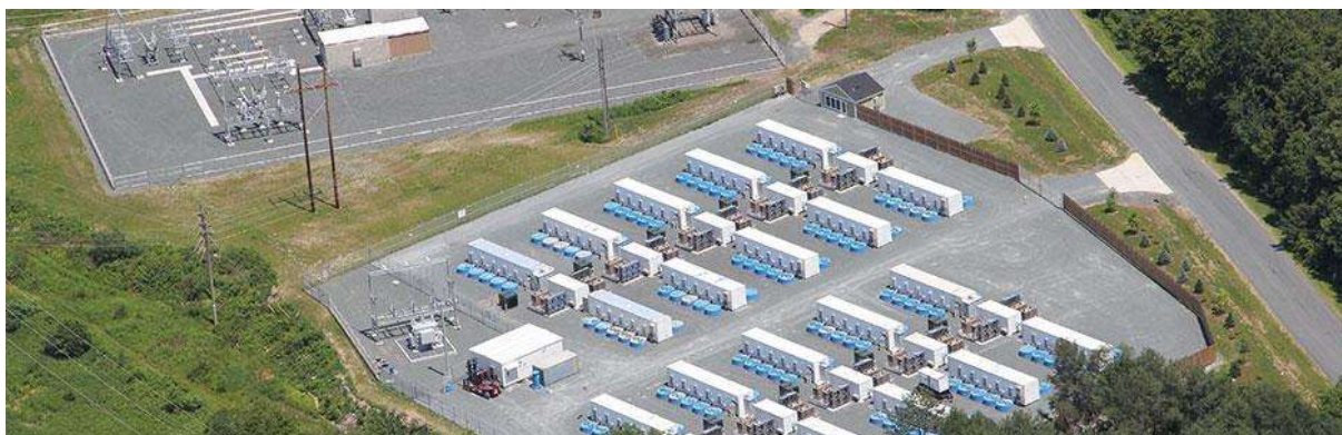
Figure 5.7 Stephentown flywheel system in New York interconnected at 115kV transmission system
